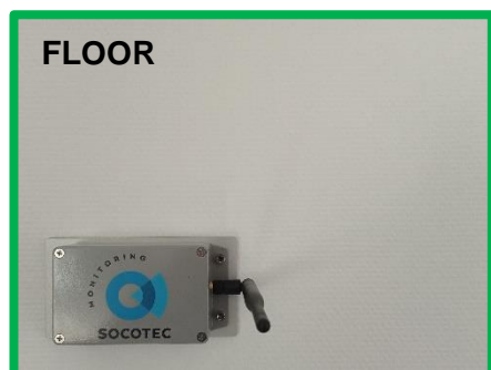
Fig.2 : good installation (above view)
