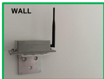
Fig.5 : good installation (front view)
