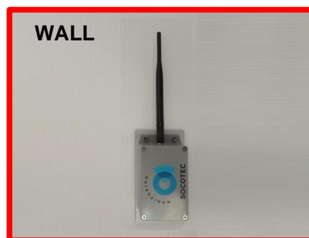
Fig.7 : bad installation (front view)
